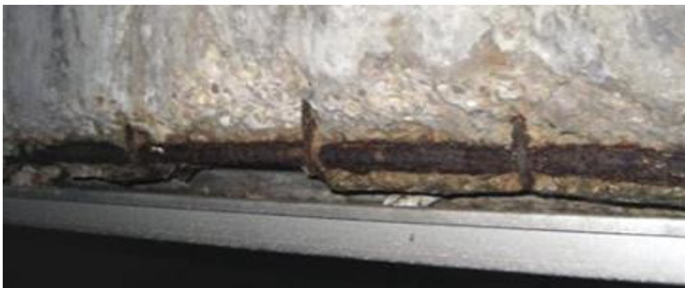
Figure 4: Typical case of concrete cover spalling
